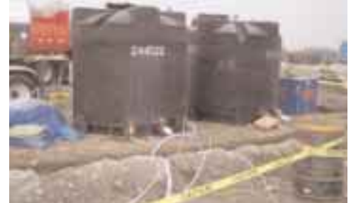
Batch tanks used to prepare injection solutions (e.g., Fe 2+ ), lines then connected to batch tanks
