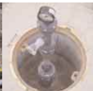
Injection well screened 30-35 ft below ground surface (BGS)
