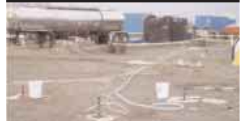
Lines carrying chemicals to injection wells
